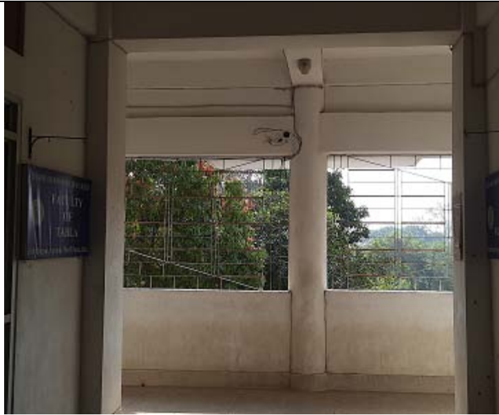
CCTV Camera installed
